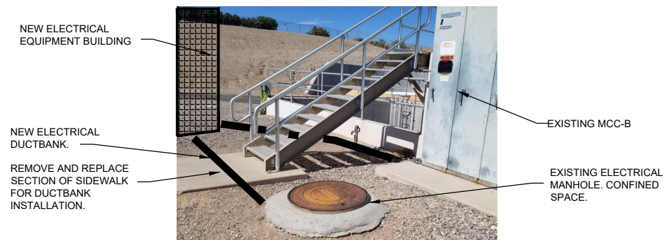
3 PHOTO 3 - ELECTRICAL MANHOLE E-402 NO SCALE
