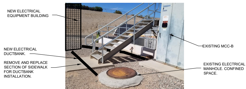
4 PHOTO 3 - ELECTRICAL MANHOLE E-501 NO SCALE
