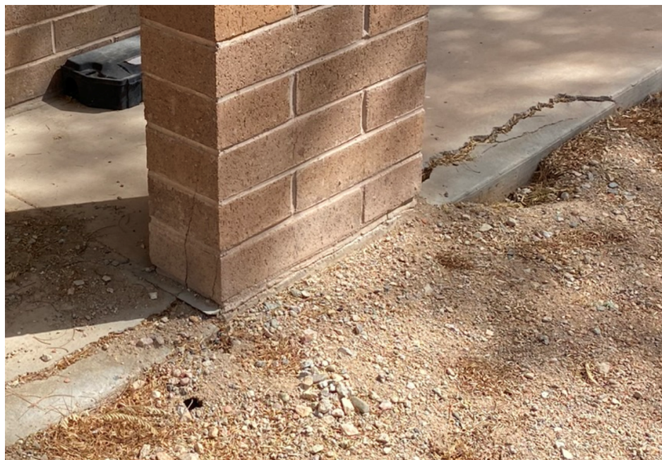
Photo 8: Close-up of column cracking
