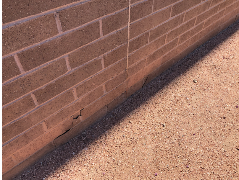
Photo 5: Typical masonry wall spalling
