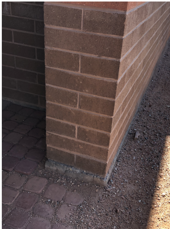
Photo 4: Masonry spalls at wall
