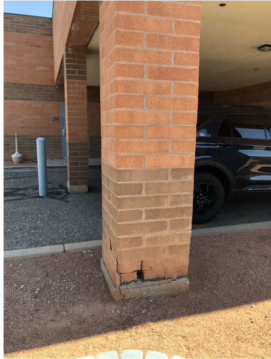
Photo 1: Front Face Exterior Deteriorated Column
