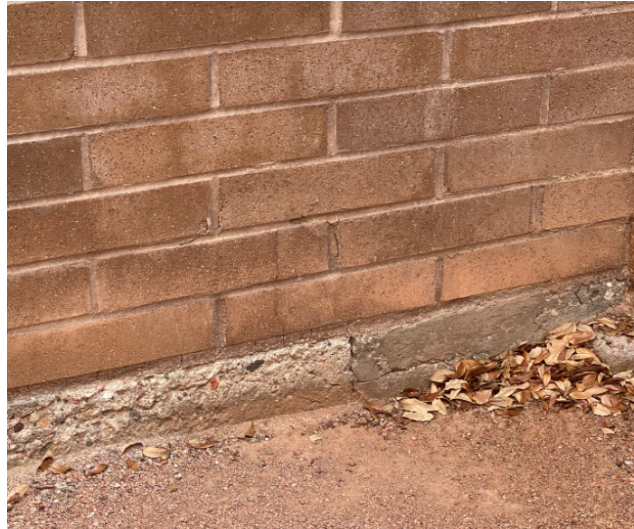
Photo 7: Close-up of masonry wall spalling & foundation deterioration
