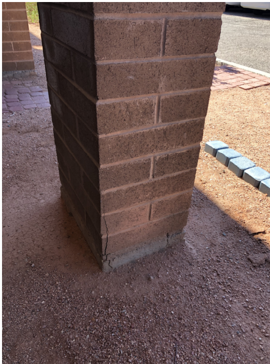
Photo 2: Rear faces of exterior deteriorated column
