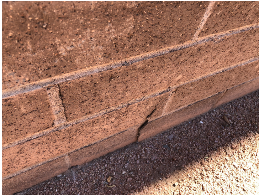
Photo 6: Close-up of masonry wall spalling
