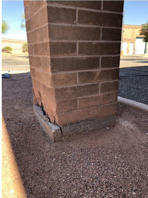
Photo 3: Close-up of exterior deteriorated column
