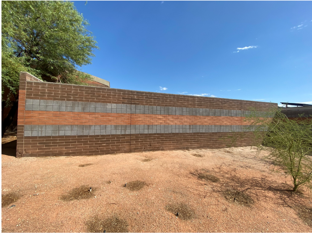
Photo 9: Site wall foundation deterioration
