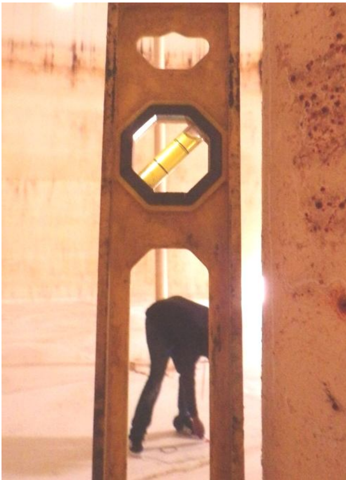
59. Center column not plumb.
