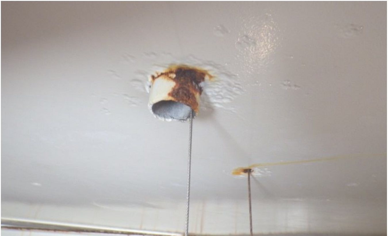
68. Corrosion around target gage equipment penetrations through roof.
