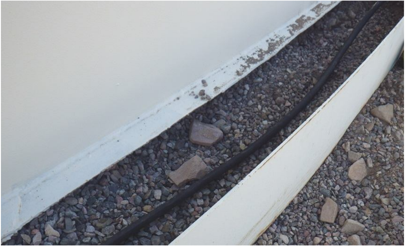
17. Bottom plate, coaxial cable, and retaining ring. Note gaps between gravel and bottom plate.
