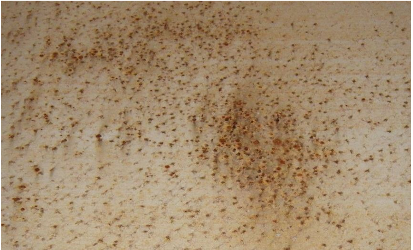
83. Blistered shell coating.
