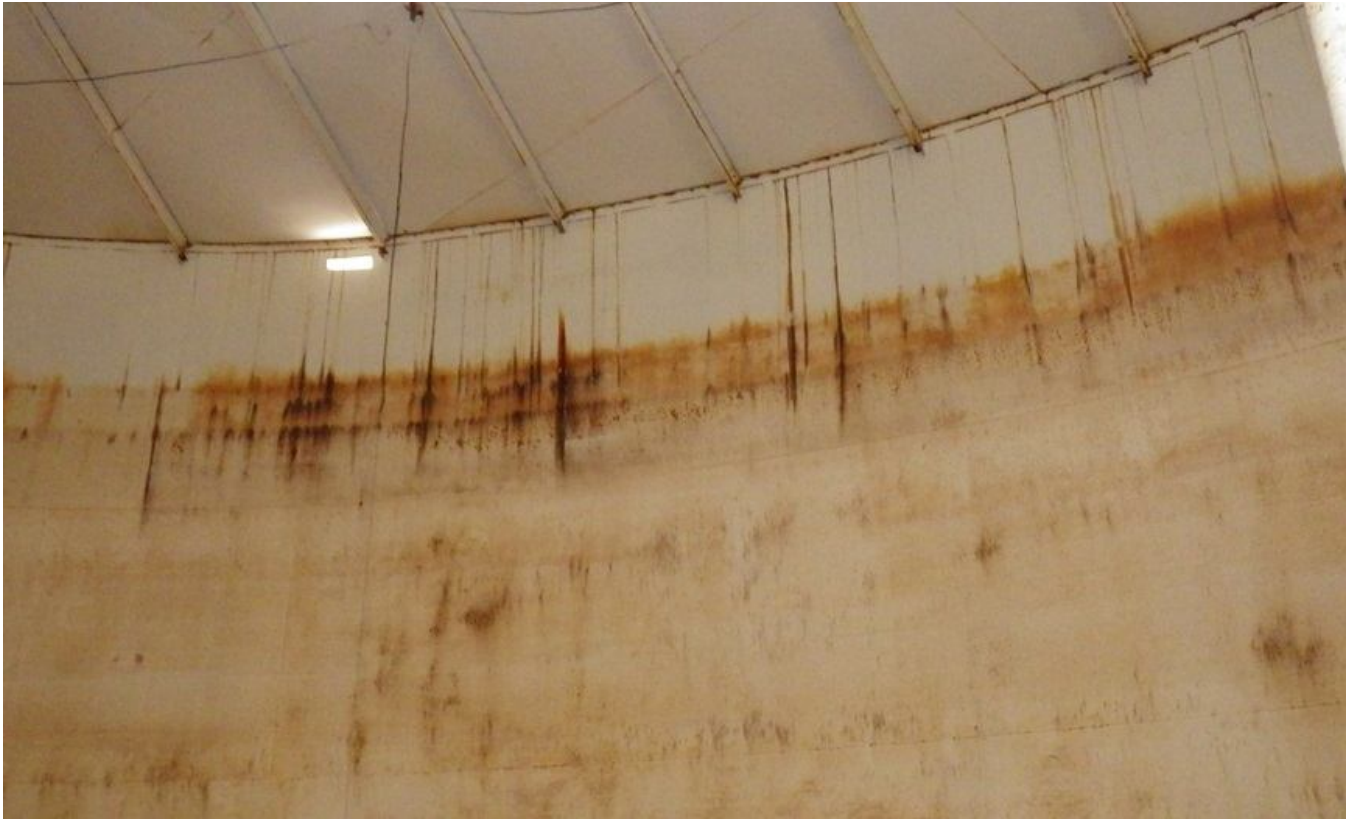
81. Corrosion on upper shell.
