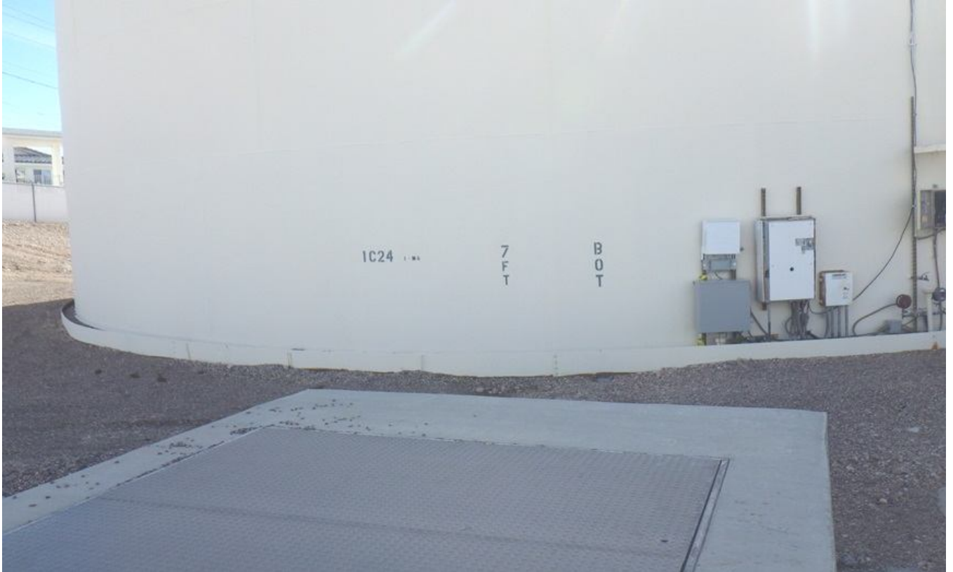
20. Valve vault exterior, information stenciled on tank, and electrical cabinets.
