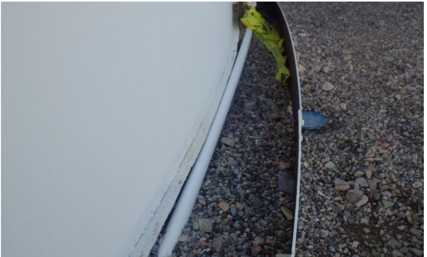
10. Retaining ring around tank. Note debris.
