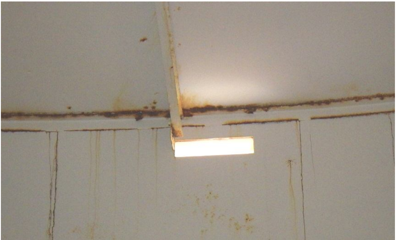
72. Corrosion and metal loss along roof-to-shell connection.
