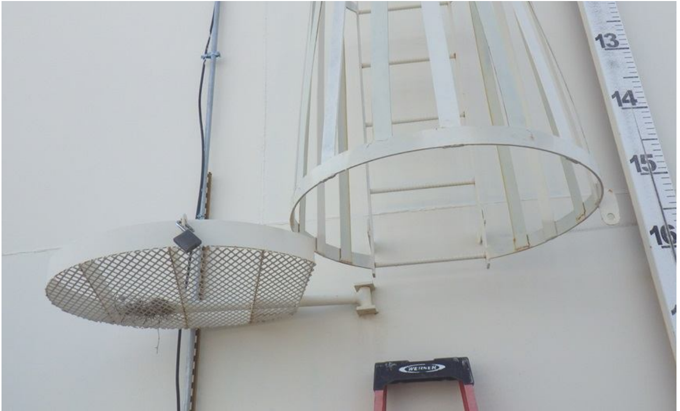
33. Vandal deterrent at base of safety cage.
