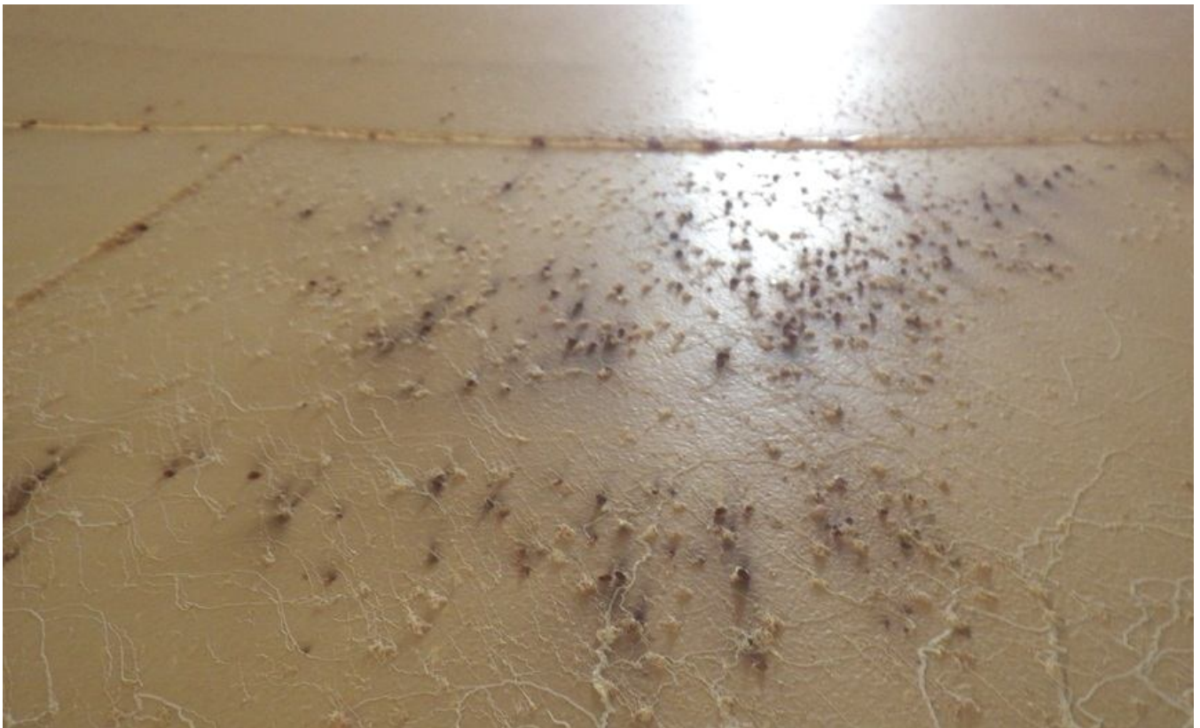
82. Blistered shell coating and hard, stringy substance on shell.
