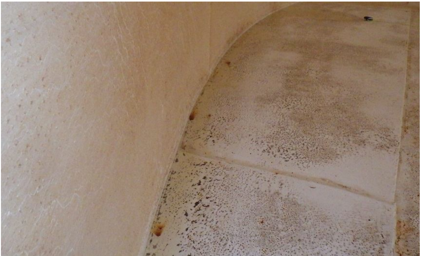
90. Corrosion and blistered coating on floor.
