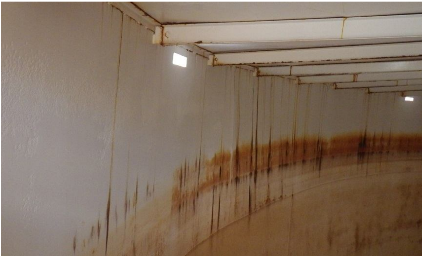
80. Corrosion on upper shell.
