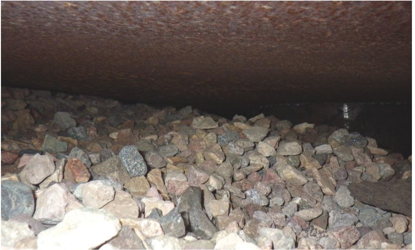
19. Corrosion on underside of bottom plate at gap.
