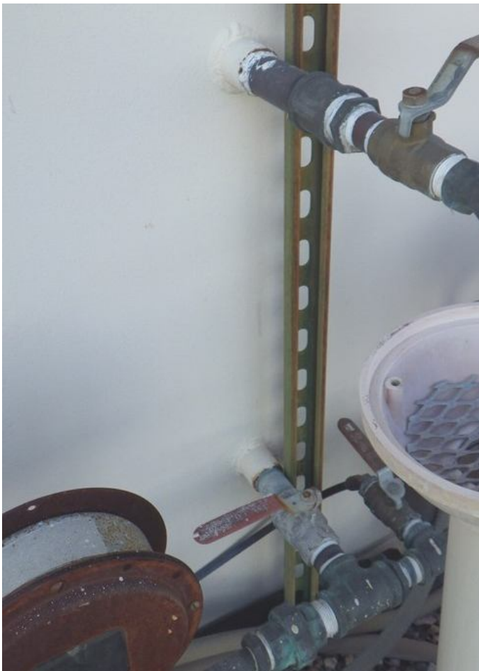
23. Coupling penetrations and valves on shell.
