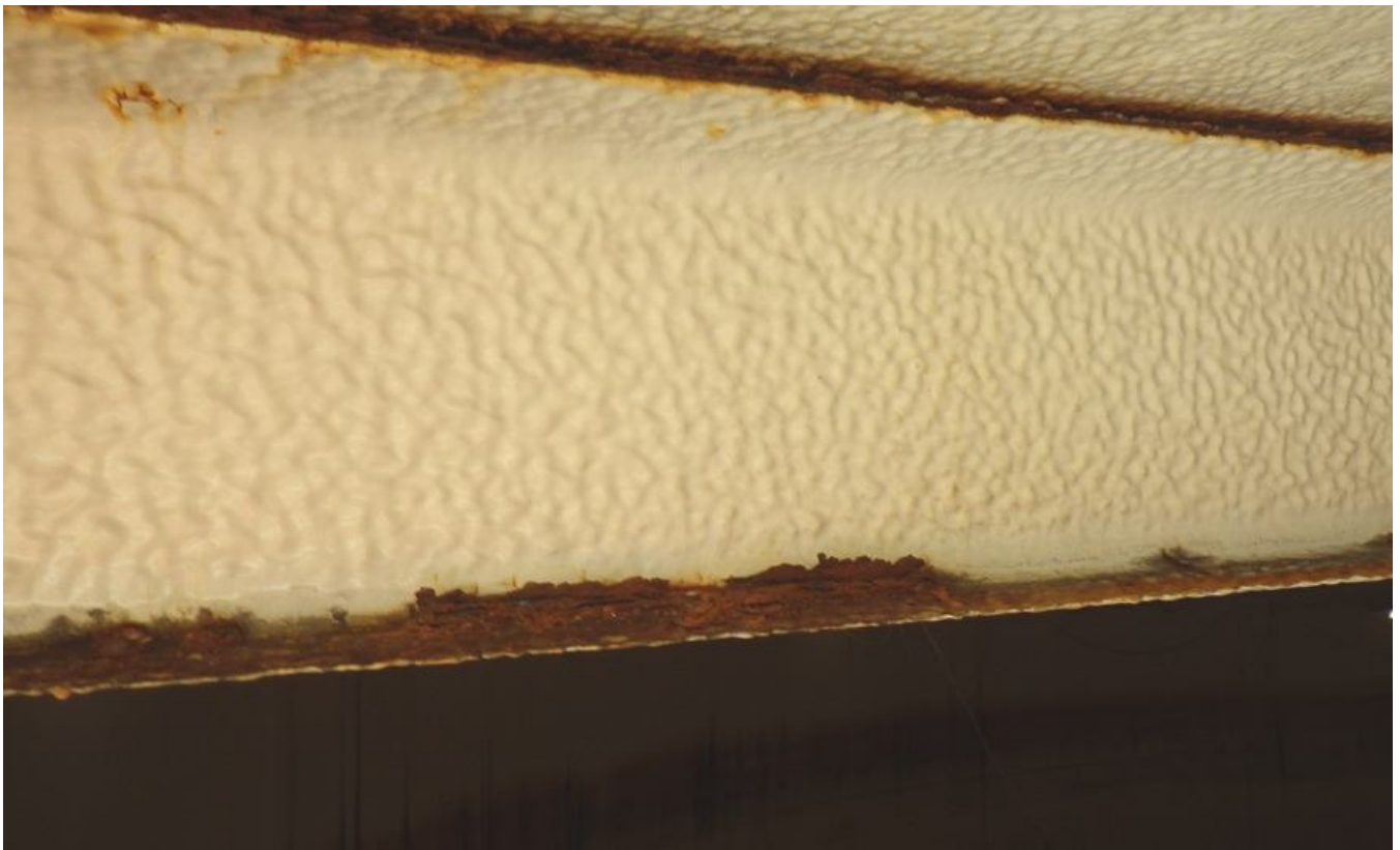
70. Corrosion and metal loss along rafter.
