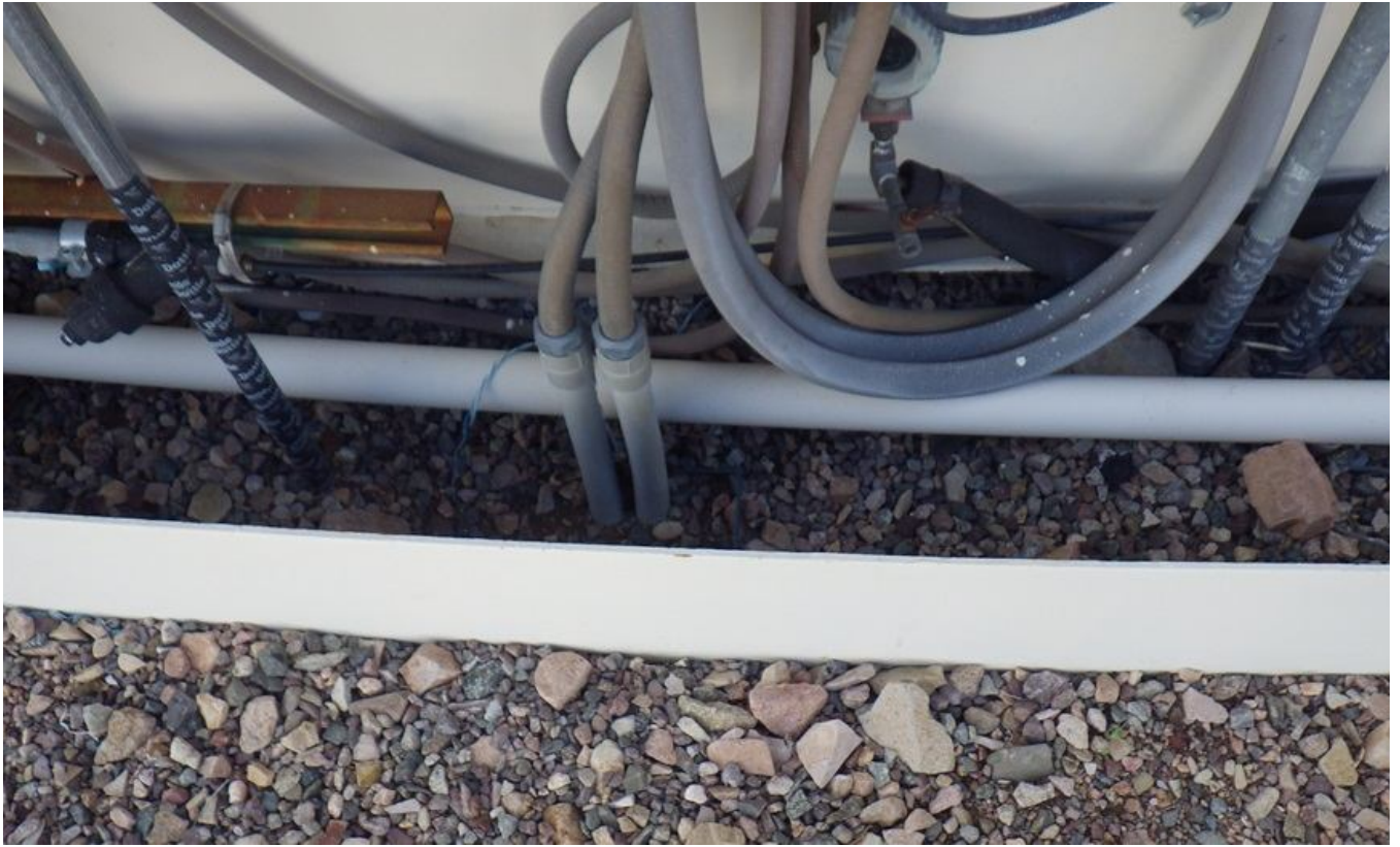
21. Electrical equipment adjacent to tank.
