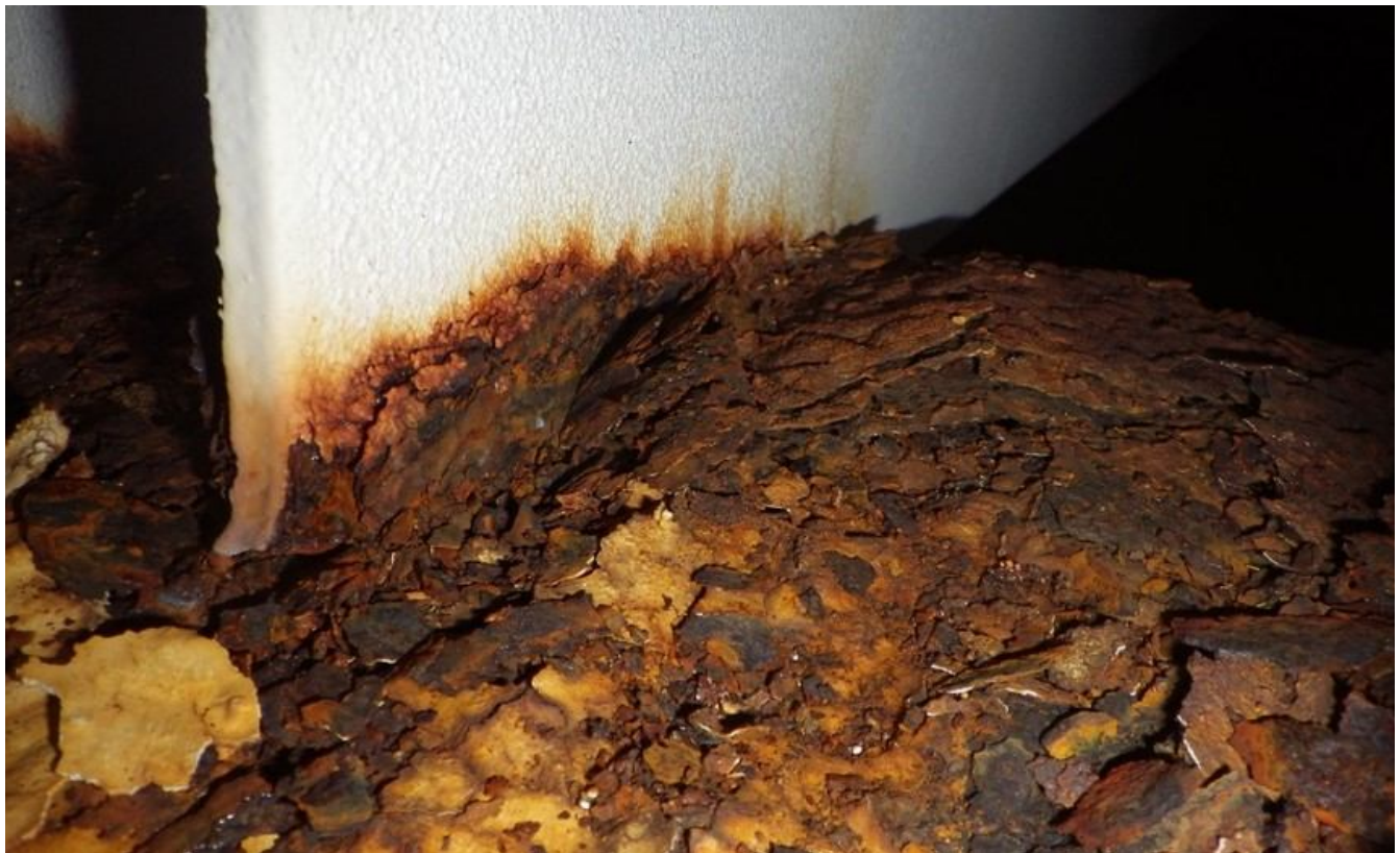
54. Corrosion and metal loss on rafter end and top side of center hub at removable cover vent.
