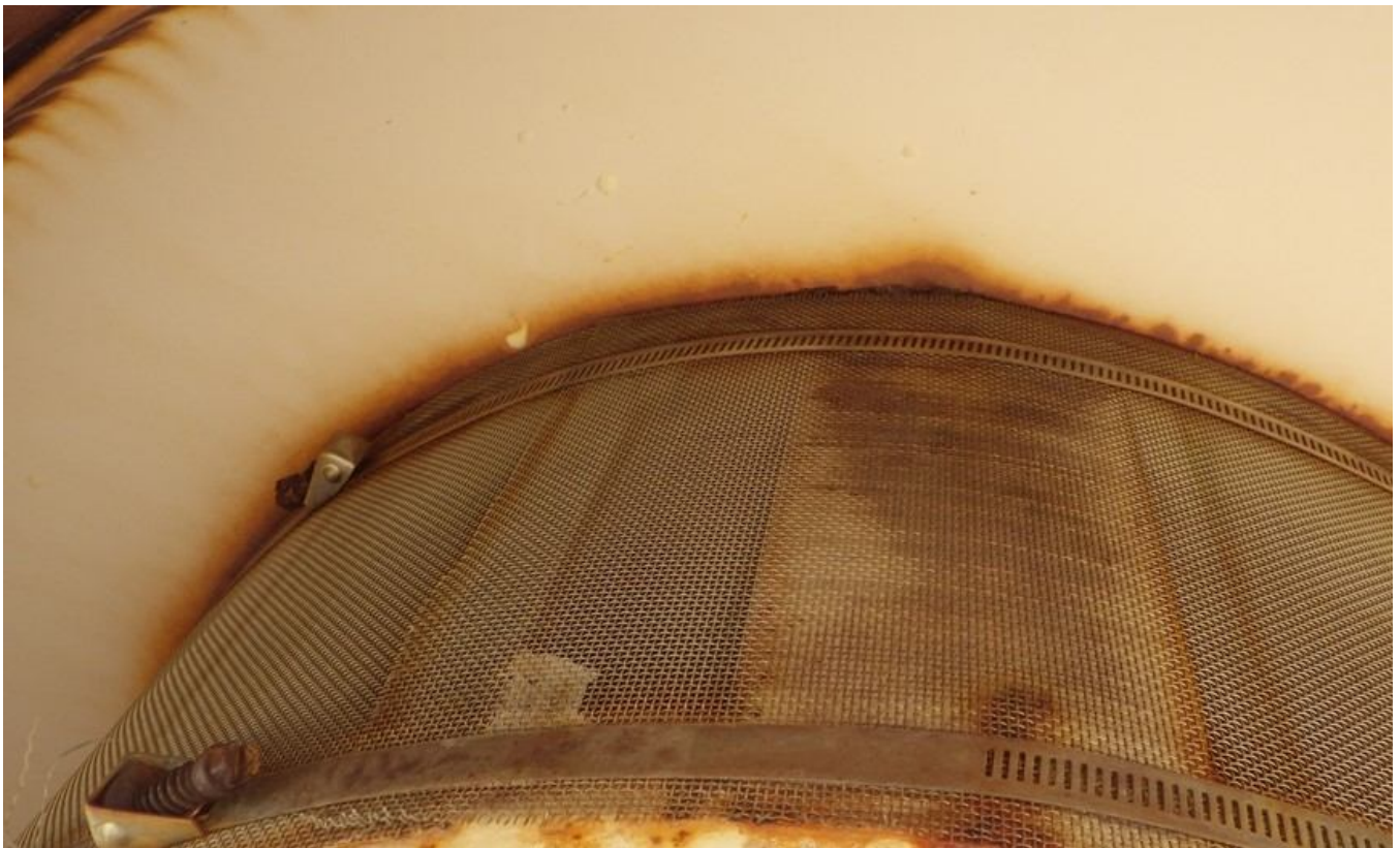
48. Corrosion on roof vent.
