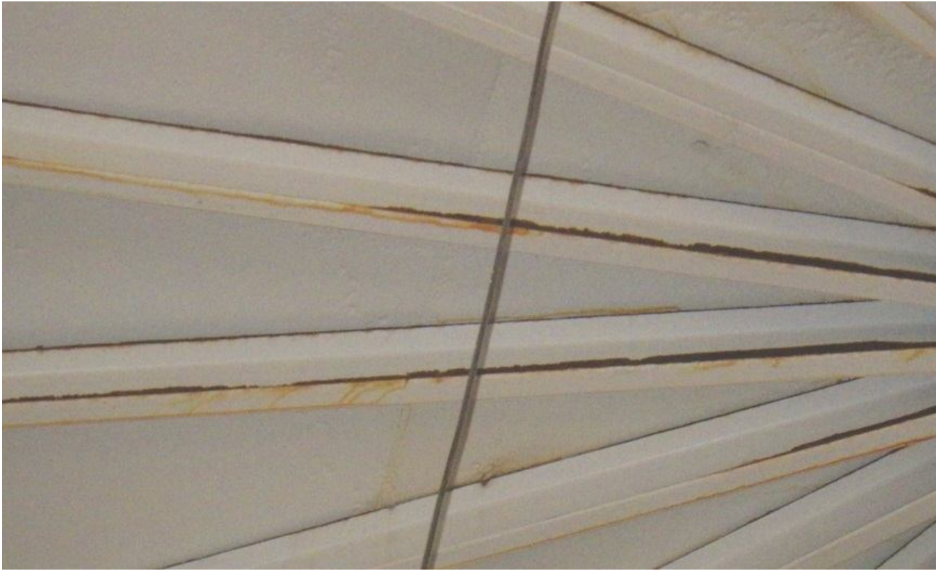
61. Corrosion on roof rafters.
