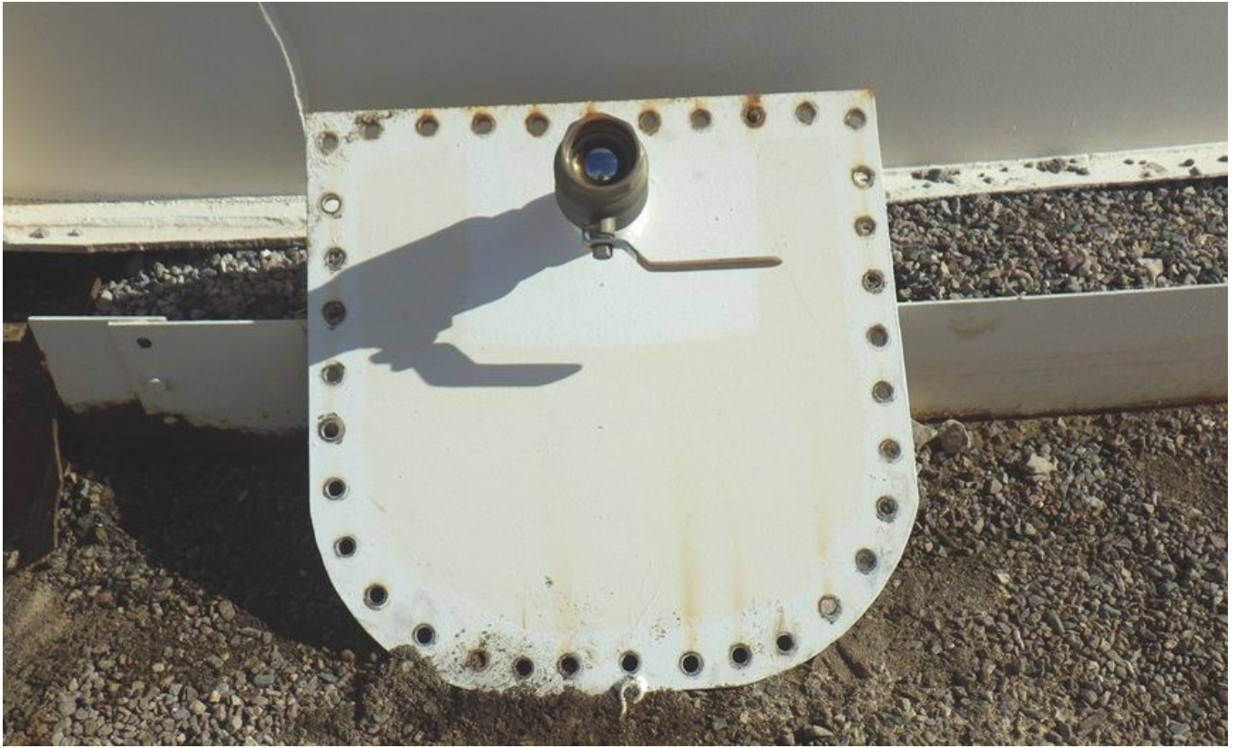
29. Coupling and valve in cleanout manhole cover.
