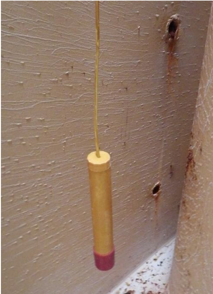
79. Cathodic protection reference electrode, coupling openings, and lower shell.
