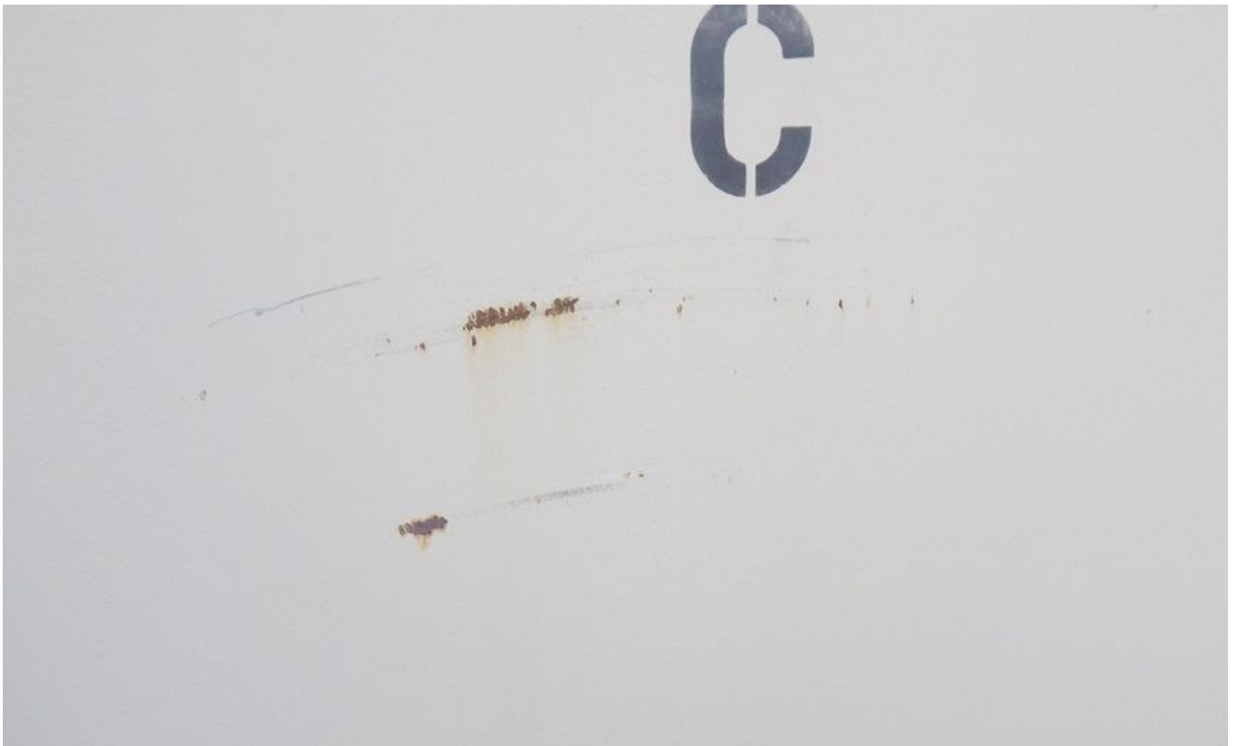
30. Corrosion and stencil on shell.
