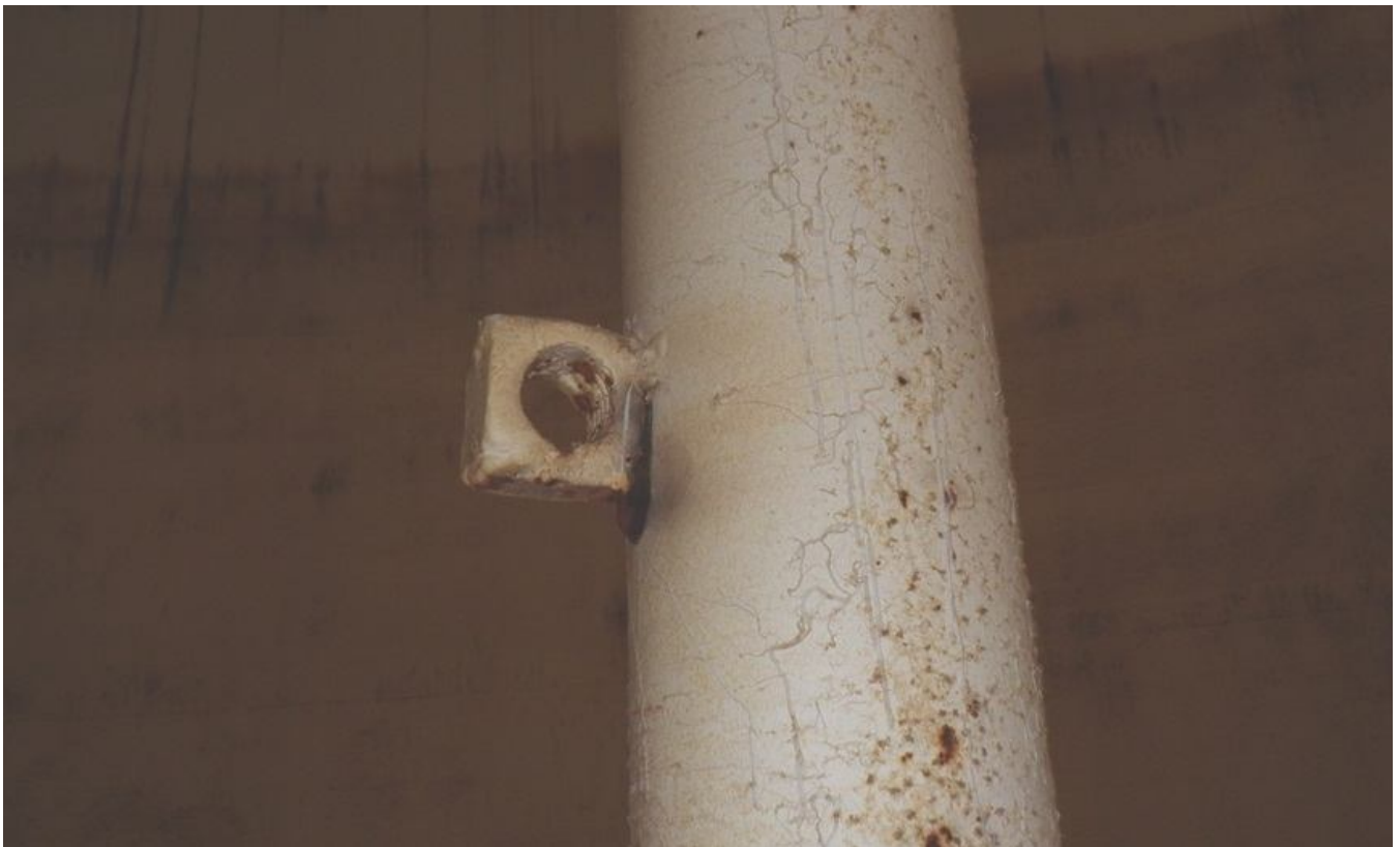
84. Blank nut and blistered coating on column.
