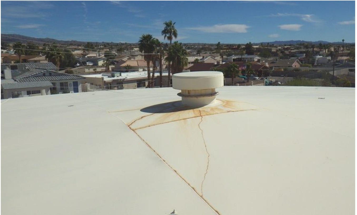
47. Rust staining on roof around vent.
