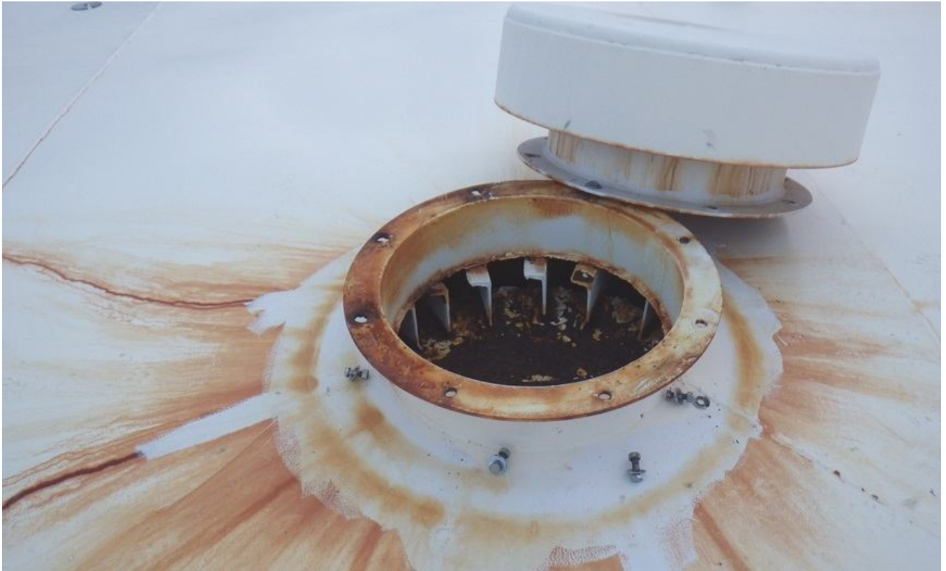
49. Corrosion within removable cover vent and rust staining on roof plates.
