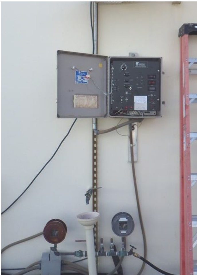
24. Cathodic protection equipment, other electrical equipment, and funnel adjacent to tank.
