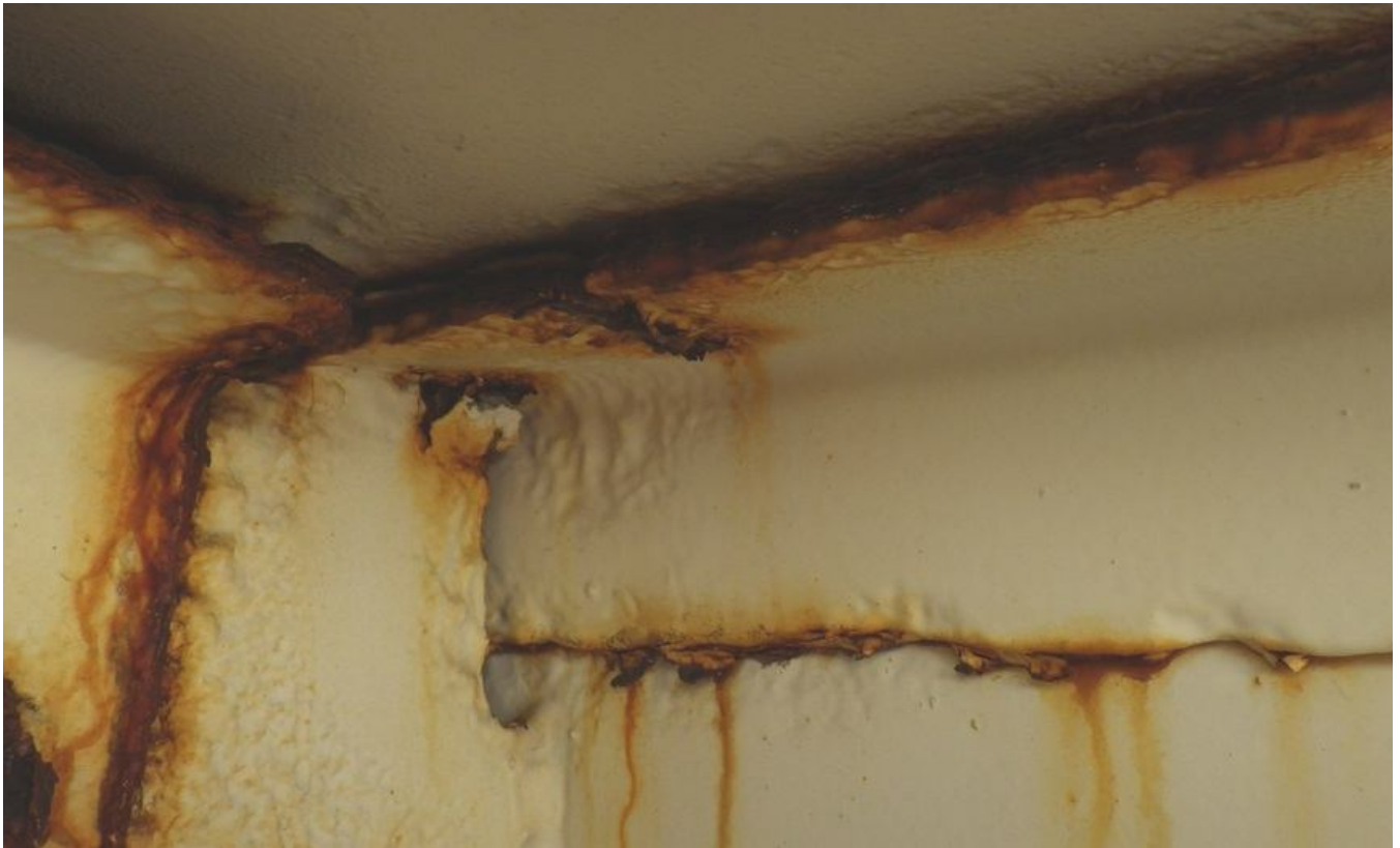
74. Corrosion and metal loss on attachment clip and along roof-to-shell connection.
