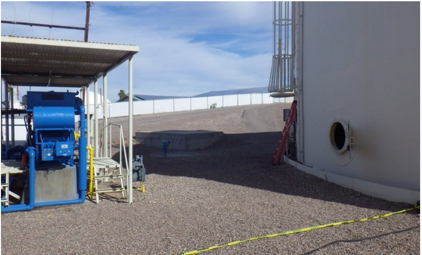
8. Pump equipment and valve vault exterior adjacent to tank.
