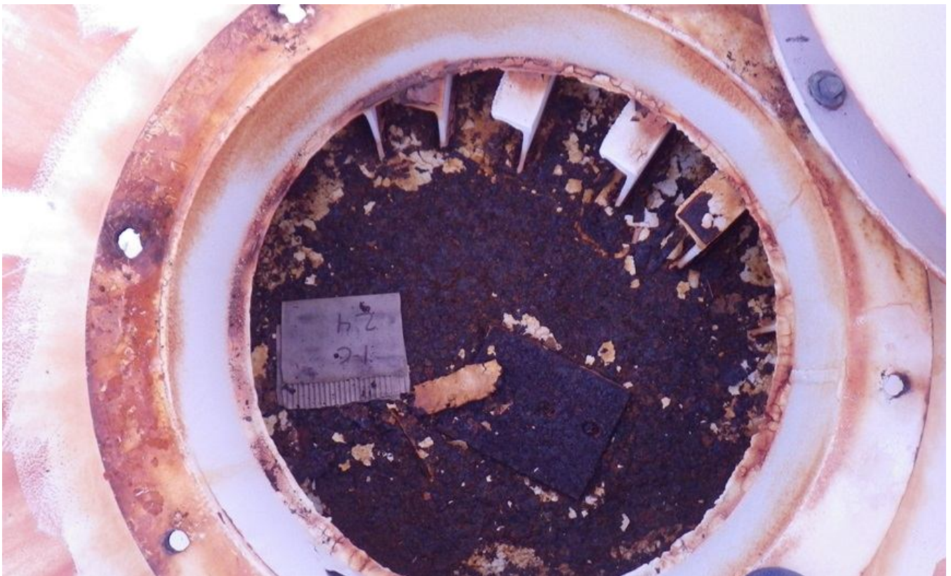
50. Corrosion and metal loss on top side of center hub at removable cover vent.
