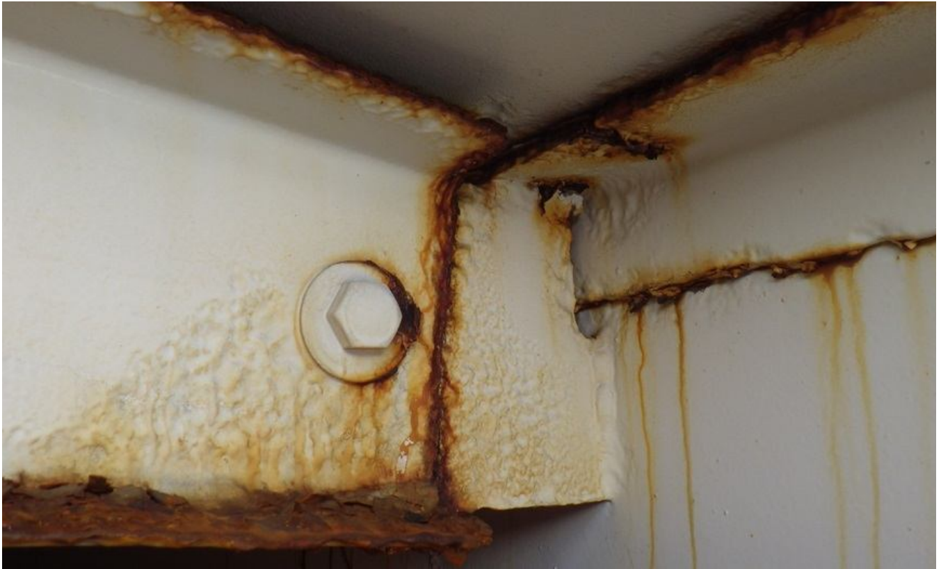
73. Corrosion and metal loss on rafter, attachment clip, bolt, and roof-to-shell connection.
