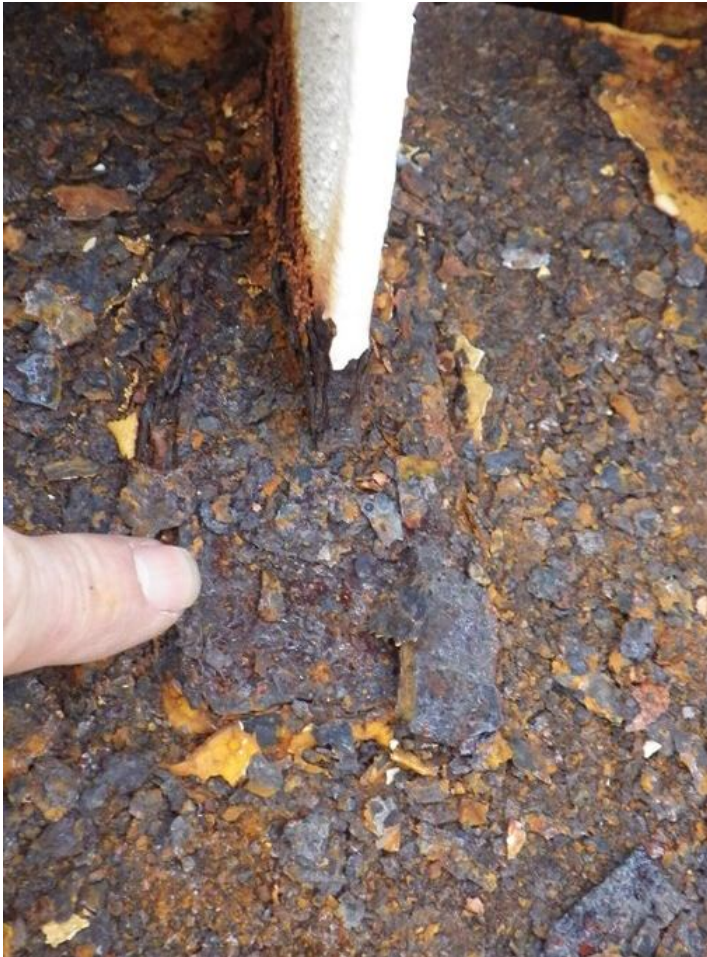
53. Corrosion and metal loss on rafter end and top side of center hub at removable cover vent.
