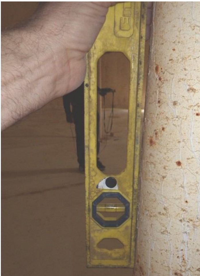
60. Center column not plumb.
