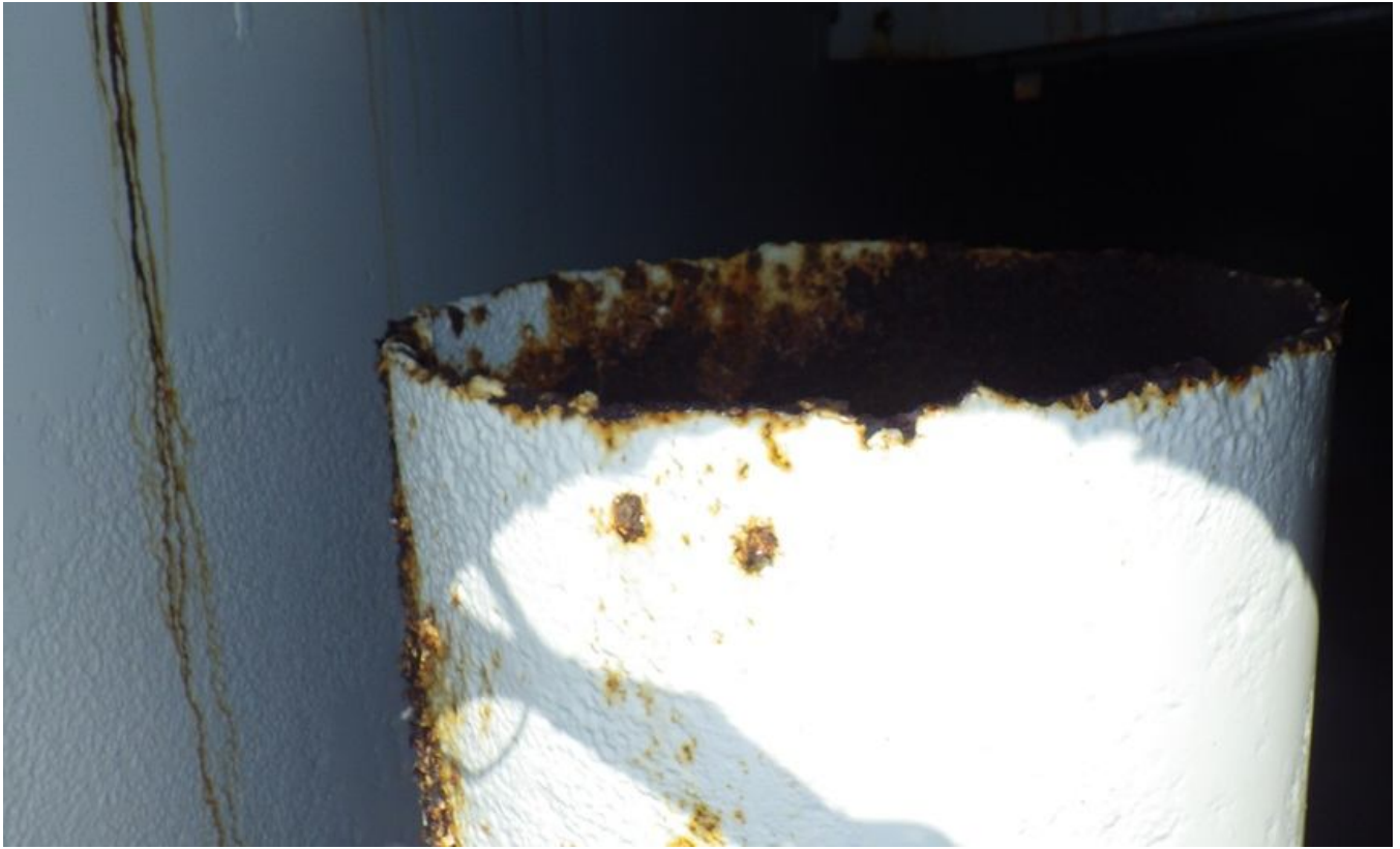
77. Corrosion and metal loss in interior overflow pipe.
