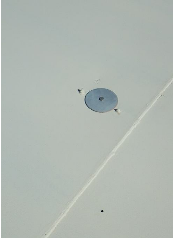
45. Cathodic protection hand hole cover plate.
