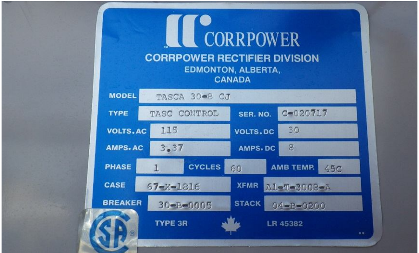
25. Cathodic protection information.
