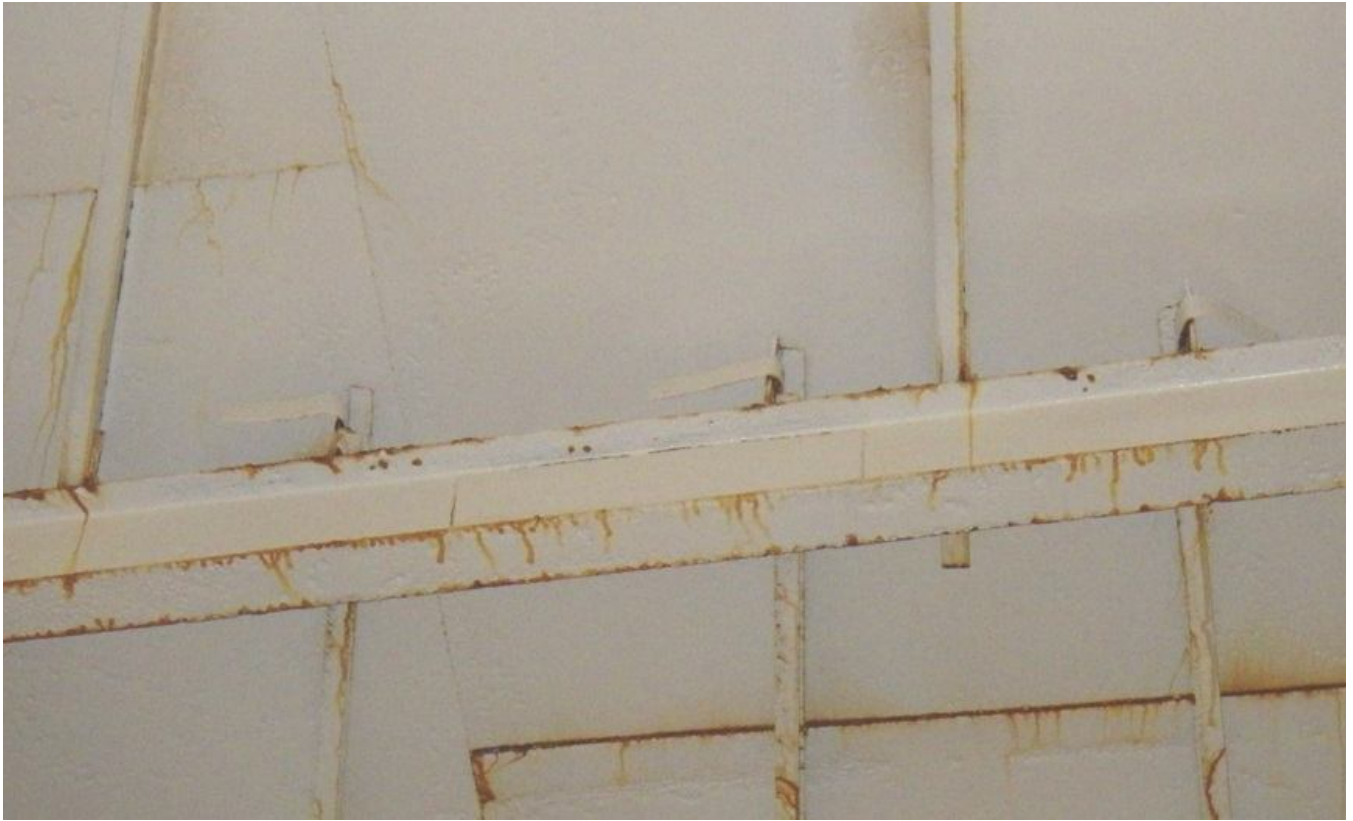
65. Unused brackets on rafter ends. Note corrosion and rust staining.
