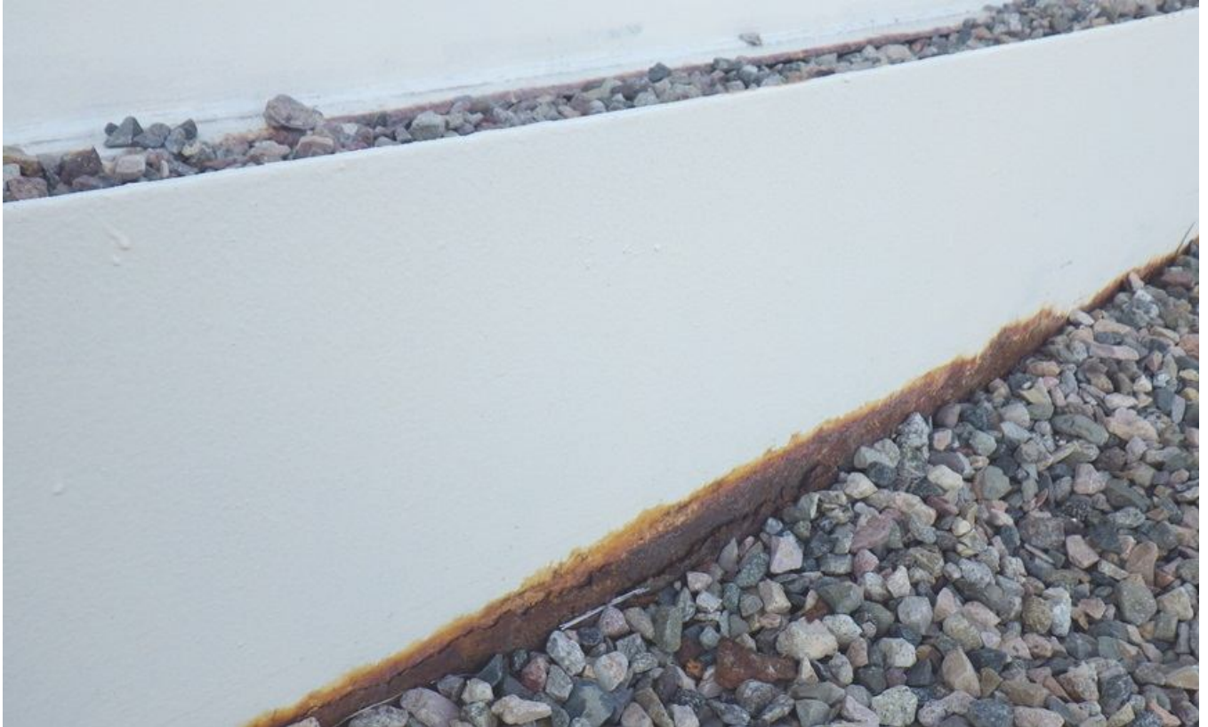
12. Corrosion and metal loss on retaining ring.
