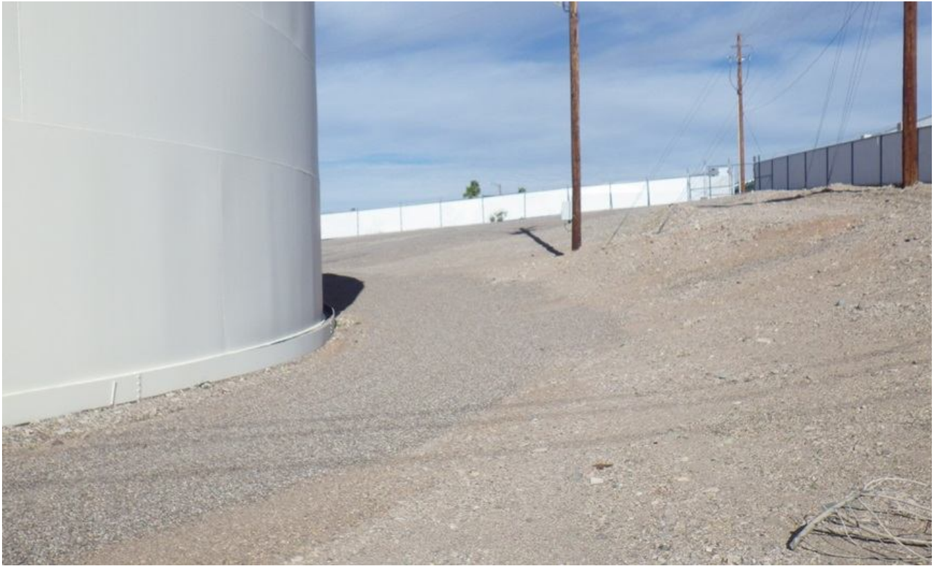
7. Site sloped toward tank.
