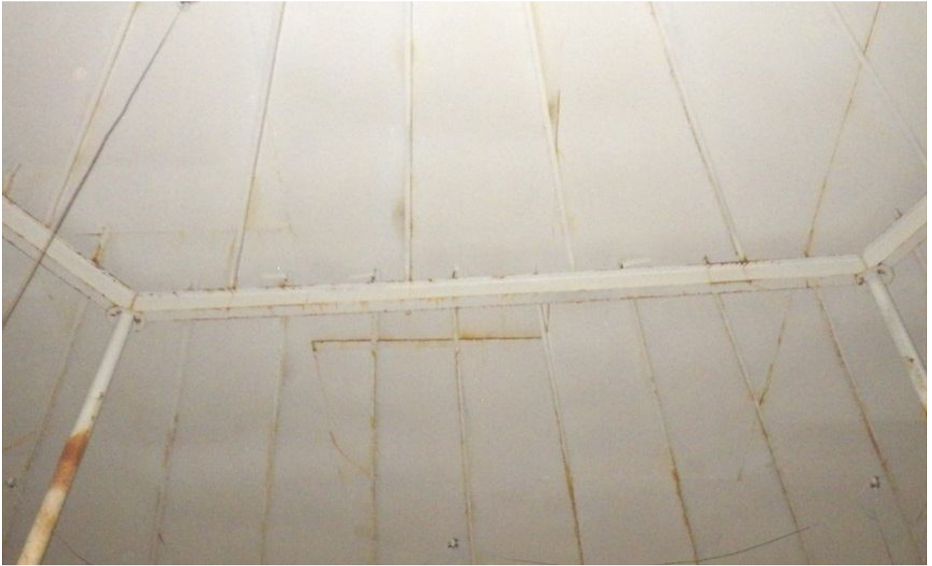
63. Outer column, roof rafters, and circumferential girder. Note corrosion and rust staining.
