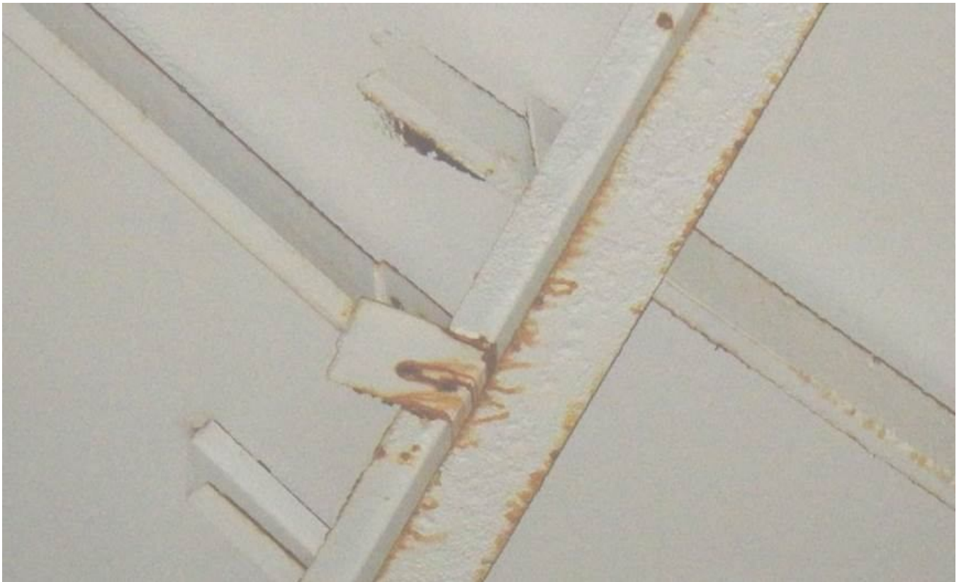
66. Unused bracket on rafter ends. Note corrosion and rust staining.
