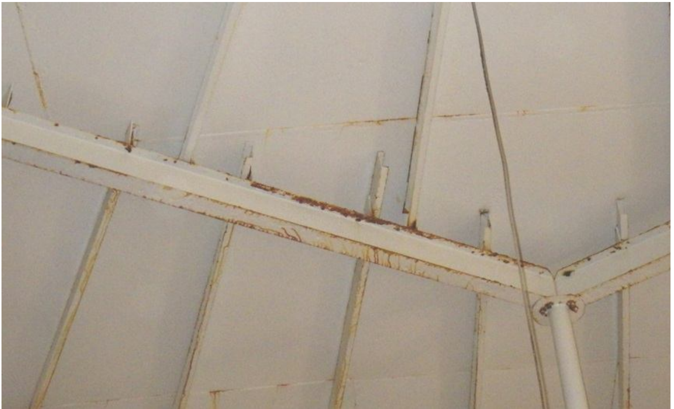
64. Outer column, roof rafters, and circumferential girder. Note corrosion and rust staining.
