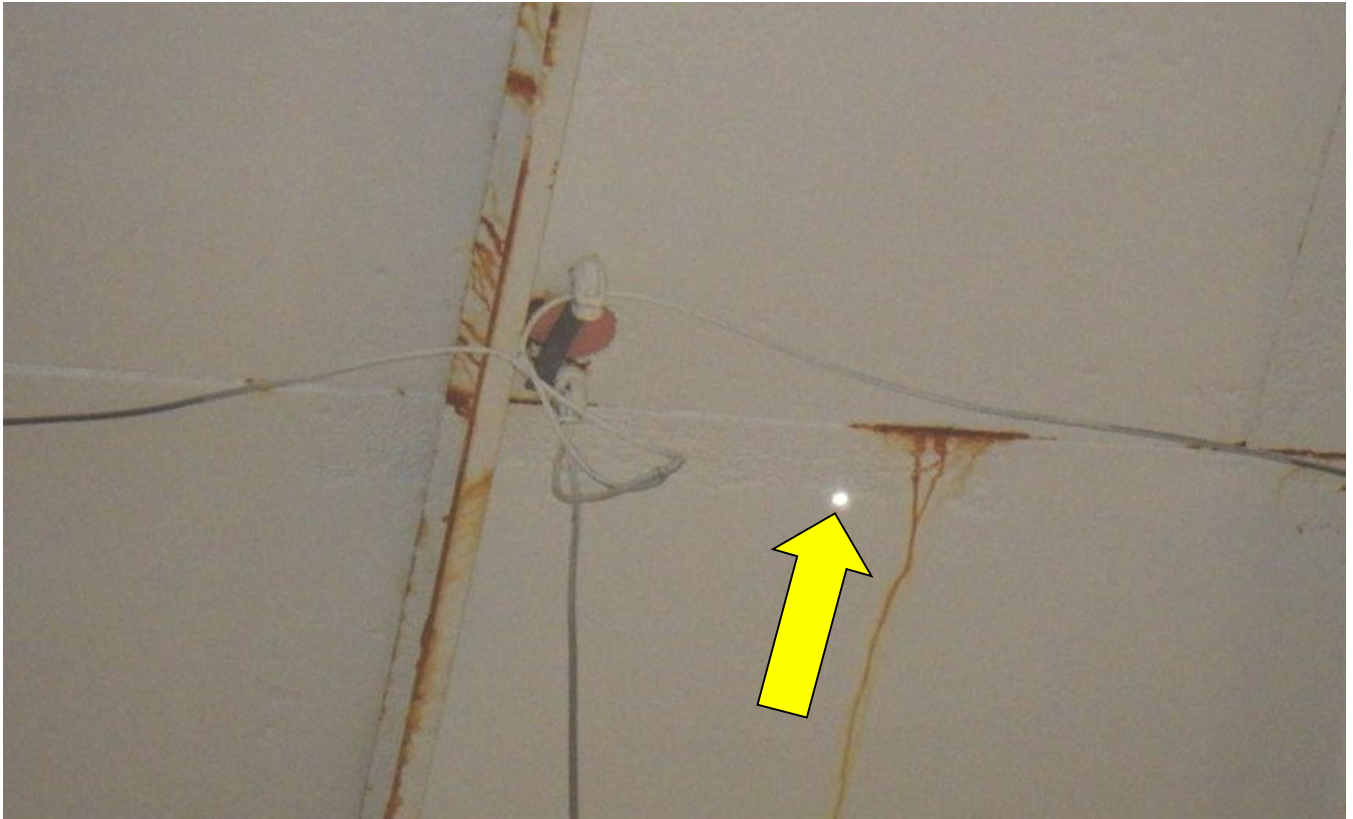
67. Cathodic protection wiring on roof and corrosion and rust staining along roof rafters and seam. Note hole in roof.
