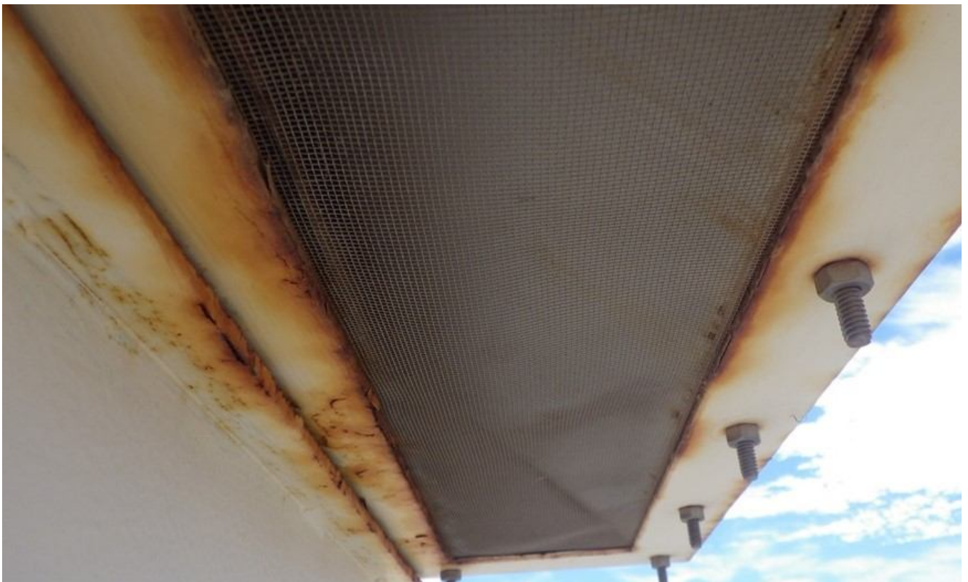
38. Corrosion on perimeter vent frame.
