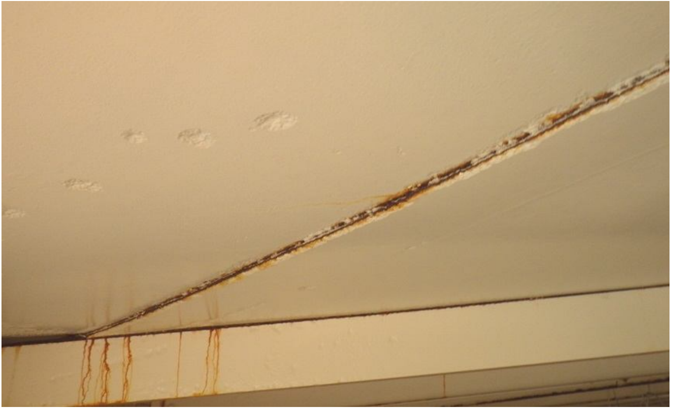
69. Corrosion and rust staining along roof plate seam and previous metal loss in roof.
