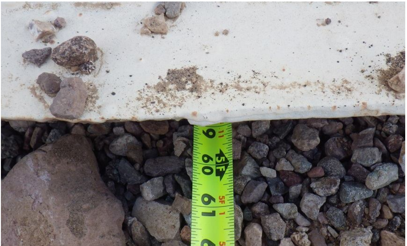
16. Gap between gravel and bottom plate.
