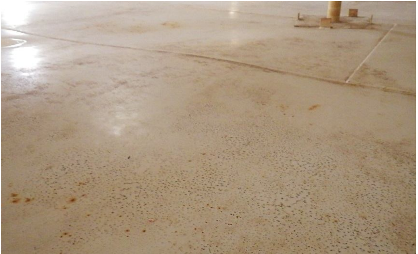
93. Irregular contour of floor. Note blistered coating and corrosion.
