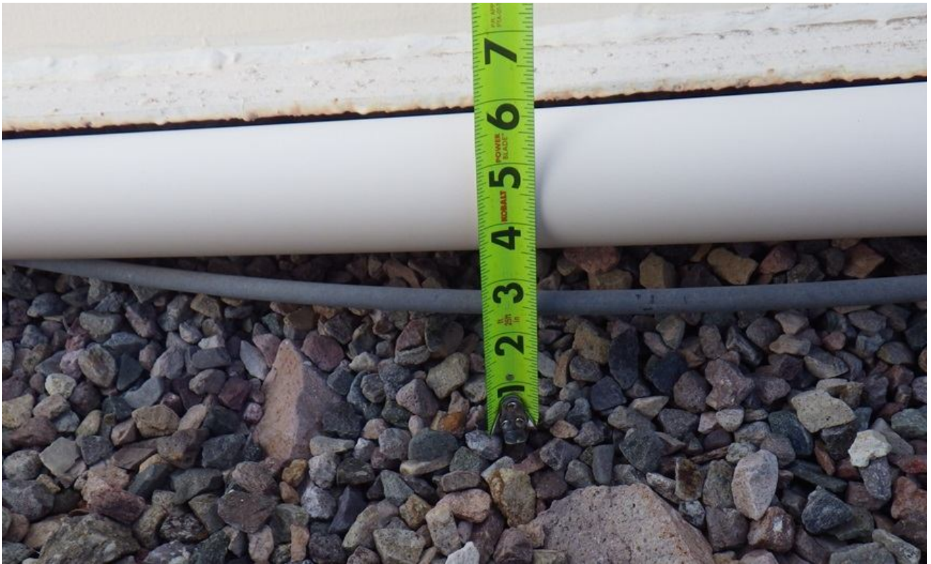
15. Conduit along gap between gravel and tank bottom.
