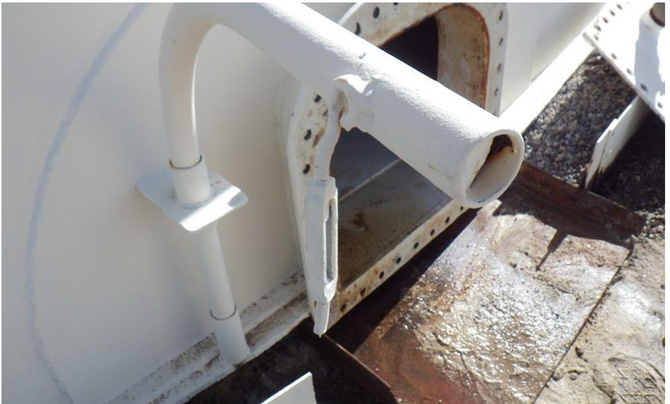
28. Broken cleanout manhole davit arm.
