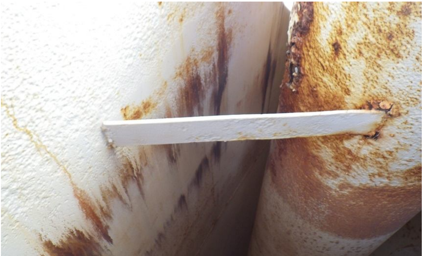
78. Corrosion in shell, overflow pipe, and bracket.
