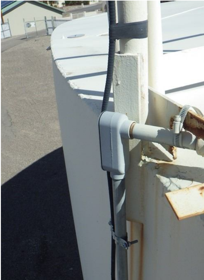
39. Conduits at shell-to-roof connection. Note conduit banded at cut-out in toe bar.
