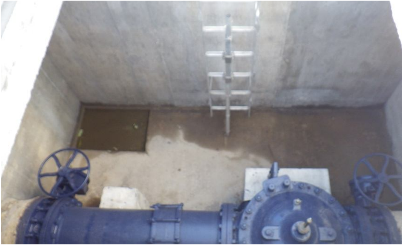
9. Valve vault interior.
