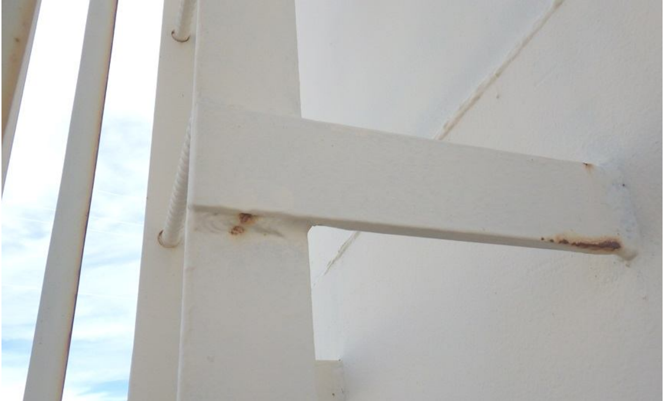
34. Corrosion at ladder bracket.
