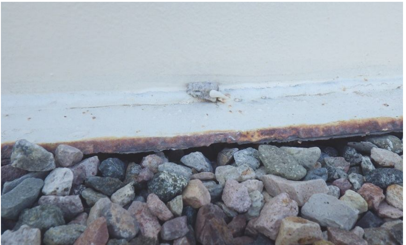
14. Corrosion and metal loss along bottom plate projection.
