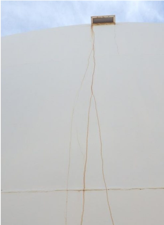
37. Rust staining streaking from perimeter vent.
