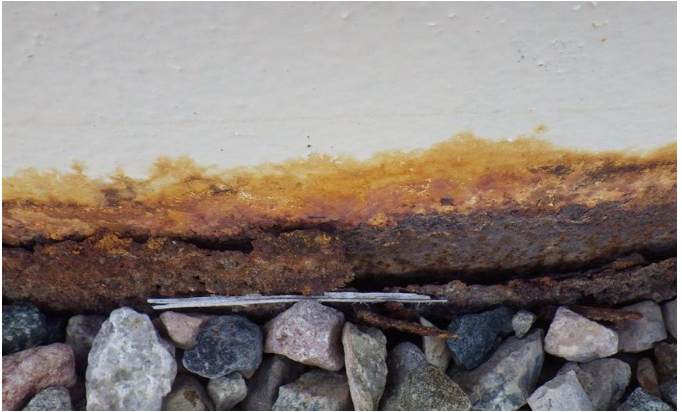
13. Corrosion and metal loss on retaining ring.
